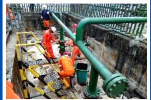
Komkom Manifold Upgrade
